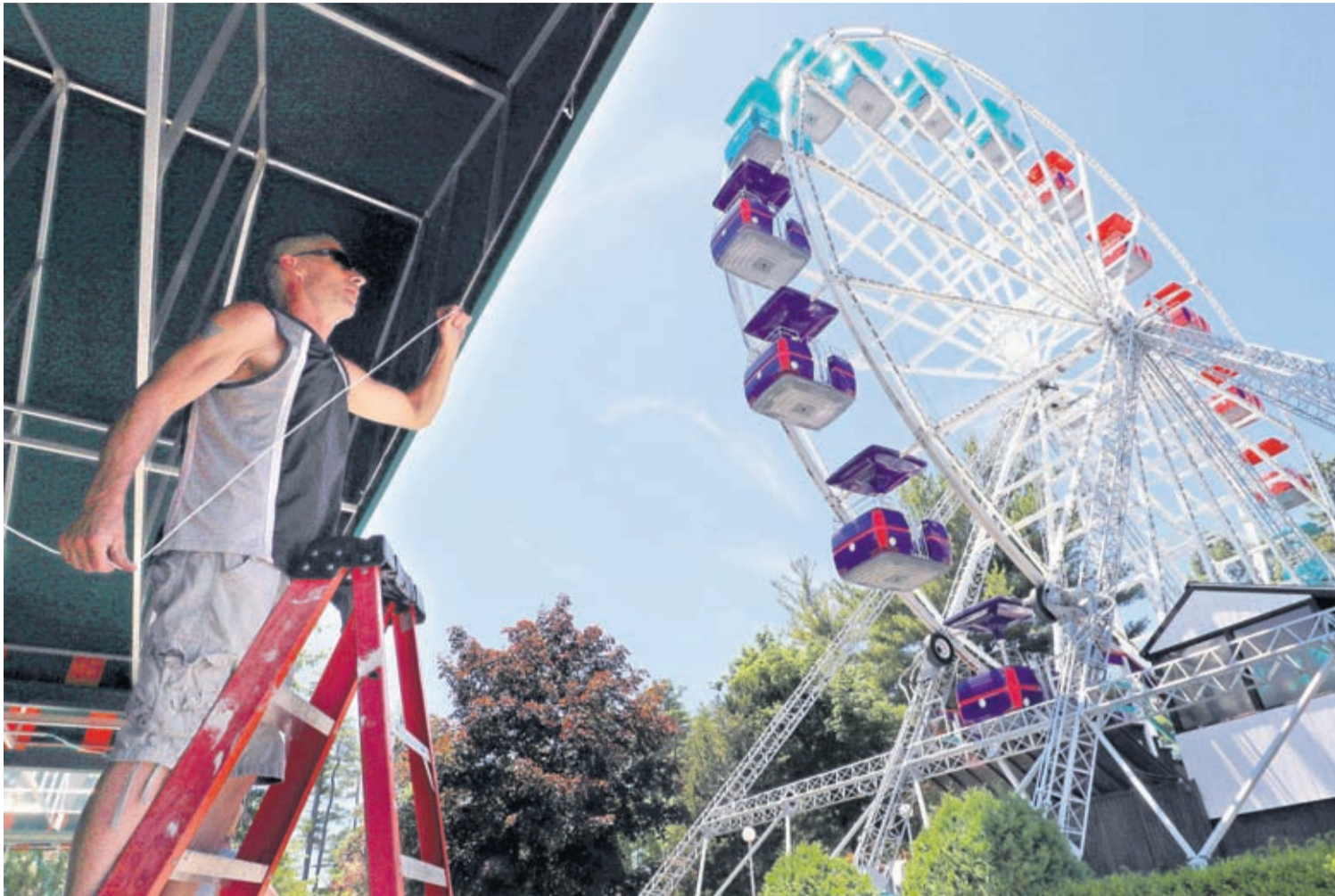
Gary Henderson installs an awning near the Giant Sky Wheel while preparing Canobie Lake Park for guests, Thursday, June 18, 2020 in Salem, New Hampshire.
